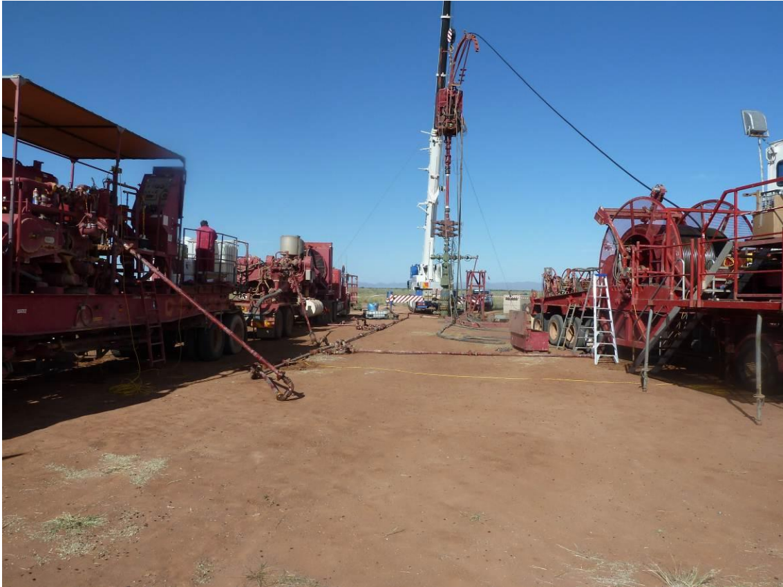
Figure 1 Recent operations at Paralana well site. Coiled tubing unit in operation (right) replacing brine fluid with water. Injection Pumps (left) set up in readiness to perform injectivity test.
